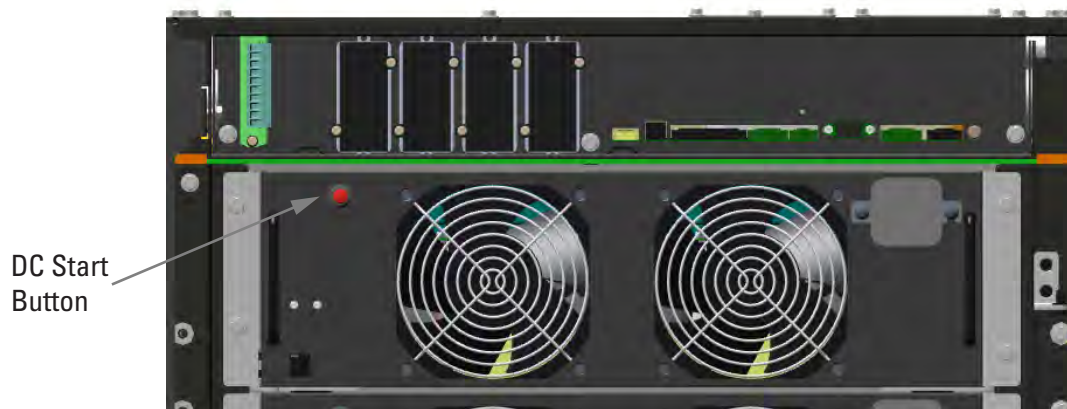
Upper Cabinet View of UPS
