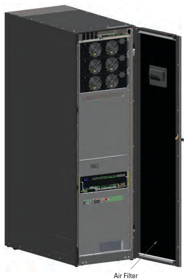
Figure 80. Air Filter Location
