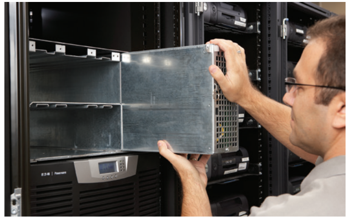
IT staff can easily install electronics modules.
