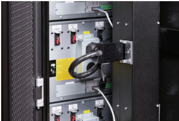
Adding modules is a simple plug-and-power procedure for IT personnel with safety-approved connectors.
