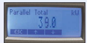
Display full system output from any UPS
