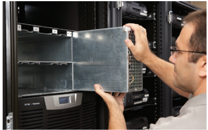
IT staff can easily install electronics modules.
