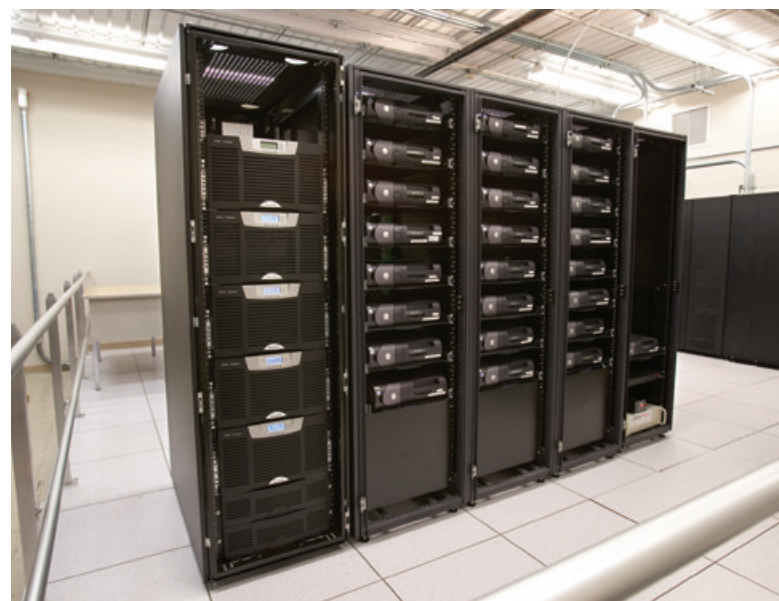
The BladeUPS remains cool even in a data center full of servers.
