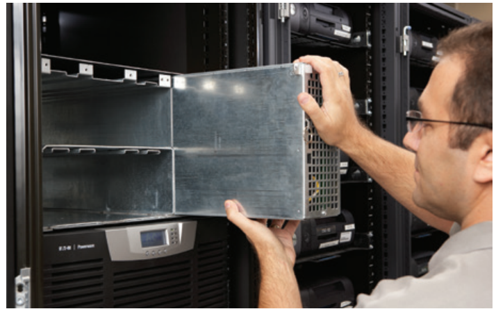
IT staff can easily install electronics modules.
