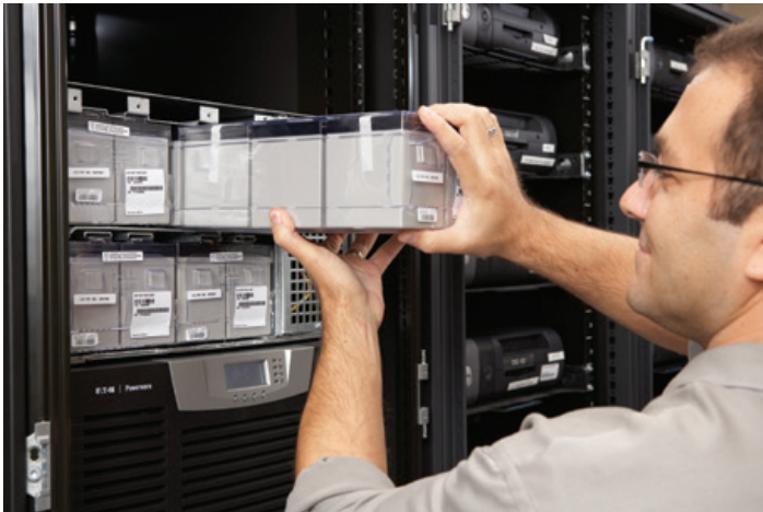
IT staff can easily replace battery modules.
