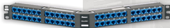
48-port, angled modular patch panel, populated with pre-terminated cassettes with UTP jack modules.
