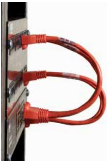
No need for horizontal cable management.
