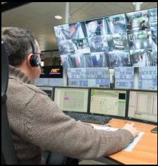
Command and Control Rooms
