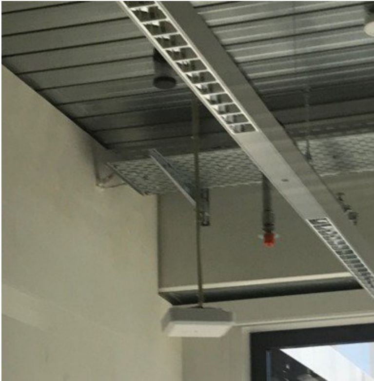
Figure 23: Example where mounting to an electrical box lowers the AP creating a more uniform cell
