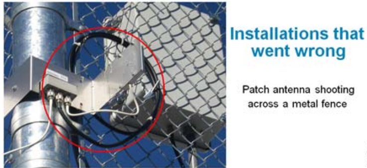
Figure 89 Patch Antenna Against a Metal Fence
