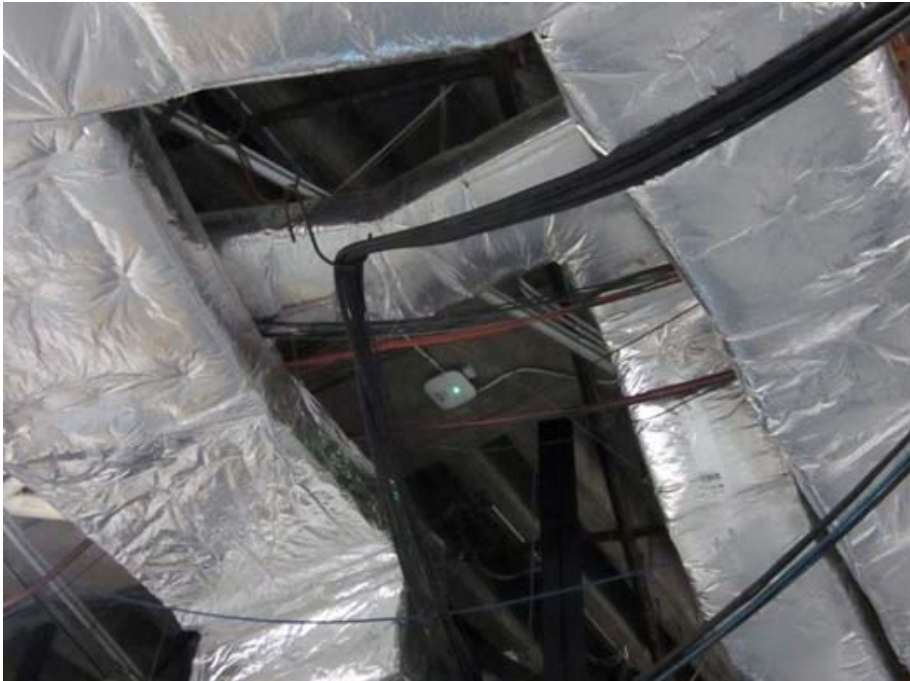
Figure 92 Example of a Poor Installation – Access Point is too High and Buried in Conductive Foil
