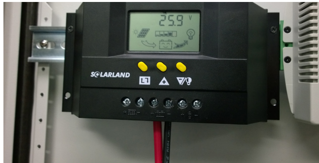
Battery Cables Connected to Controller Battery Terminals
