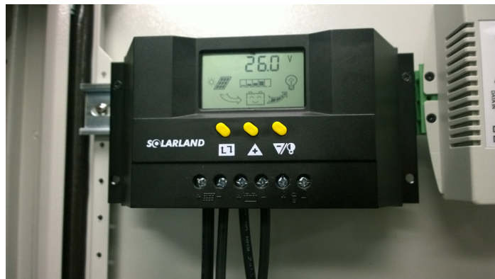
Solar Panel Cables Connected to Solar Load Terminals on Controller
