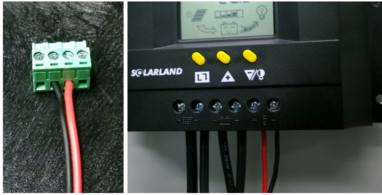
Red and Black Cable Connected Green Terminal Connector, left, and to Load Terminals on Controller, right.
