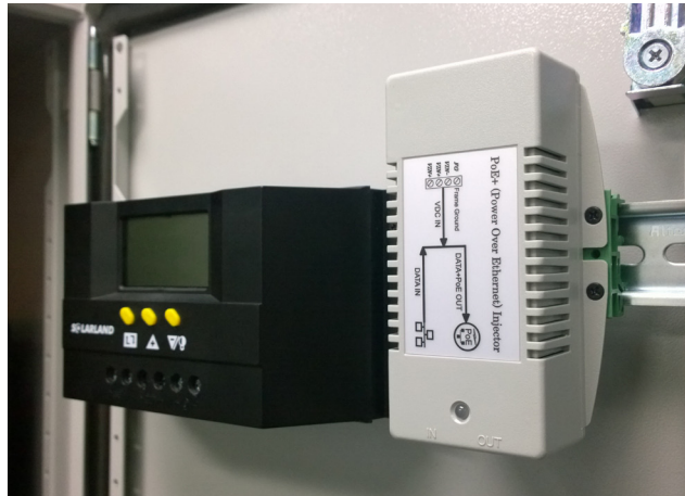
Controller and Power Injector Mounted on DIN Rail
