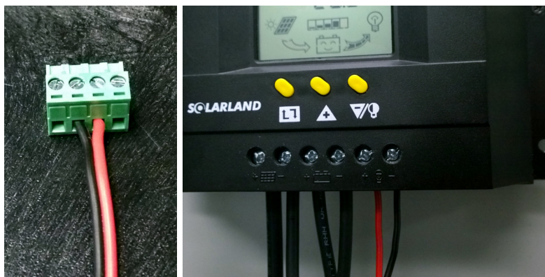
Red and Black Cable Connected Green Terminal Connector, left, and to Load Terminals on Controller, right.
