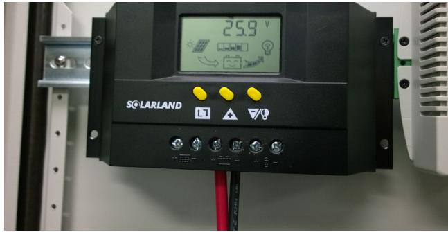
Battery Cables Connected to Controller Battery Terminals
