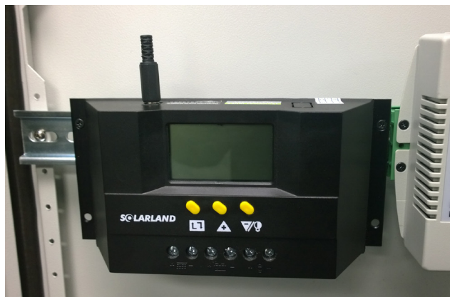
Thermal Sensor Plugged into Controller
