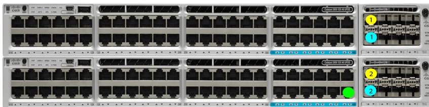
Dual 10/25GE ToR Switches (standalone or stacked)
