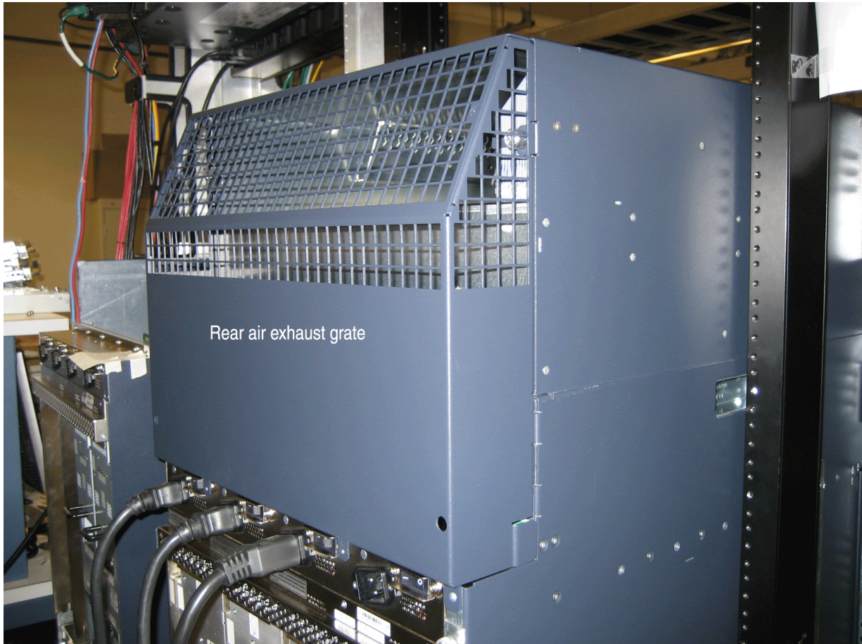
Figure 79: Extended Cable Manager (Rear View)
